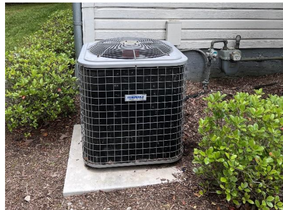
Photo 26: Unit 2 Condensing Unit
