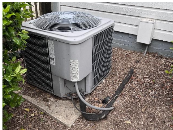
Photo 23: Unit 1 Condensing Unit
