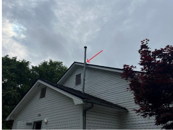
Photo 24: Loose Vent Pipe
