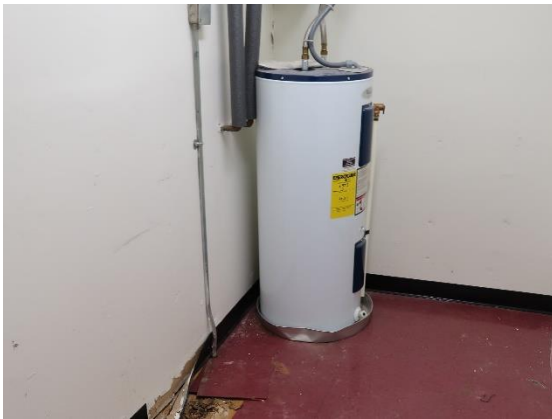
Photo 27: Domestic Water Heater
