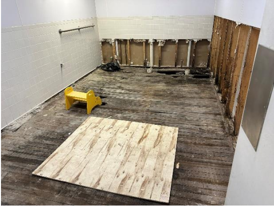
Photo 17: Water Damage in Restroom
