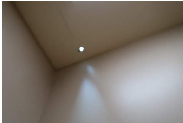
Photo 19: Hole in Ceiling Adjacent to the Kitchen Area
