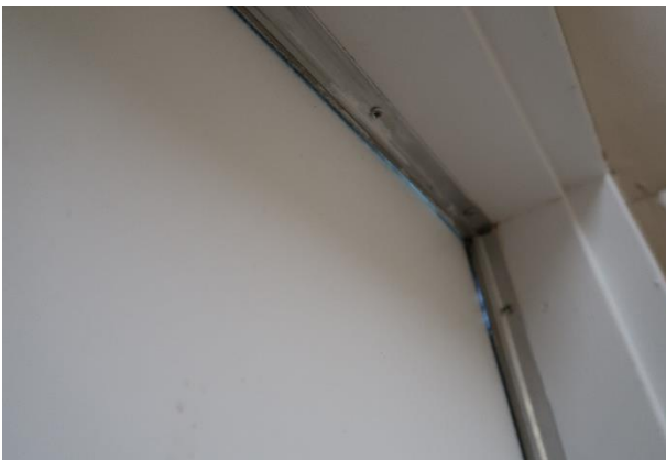
Photo 20: Gap in Weatherstripping at Rear Entrance
