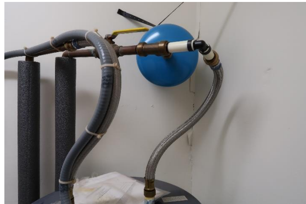
Photo 28: Domestic Water Heater Expansion Tank
