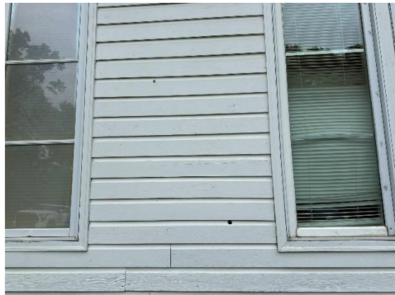
Photo 16: Hole in Siding on West Side of Building
