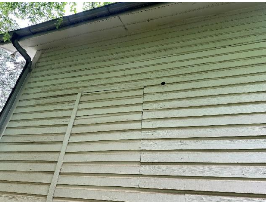
Photo 15: Hole in Siding on East Side of Building
