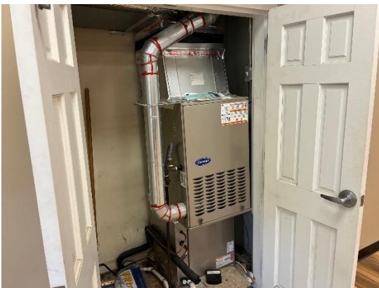
Photo 22: Unit 1 Indoor Unit
