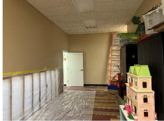
Photo 18: Wall Damage due to Water Leak in Restroom
